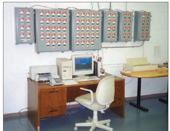
Phoenix Plaza energy manager's monitoring station where data from the facility's 80 submeters are input into energy analysis software for cost allocation and tenant billing.
