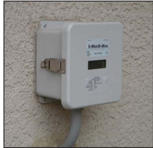
Simple, clean installation of the E-Mon D-Mon outdoor meter blends well with the housing exterior. Hondo Electric's Steve Shoop noted that "by using the E-Mon D-Mon meters with split-core sensors, installation took an average of one and a half hours per house and required minimal drywall repair and paint touch-up."
